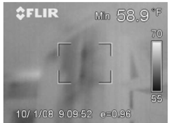
Closet interior wall is open to the attic. Could be sealed from the attic or the interior walls blown tight with densely packed cellulose insulation.
