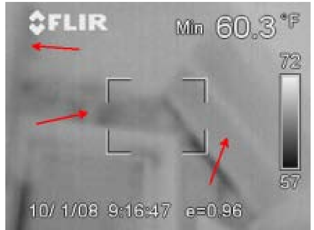
Shows leaks to the outside
