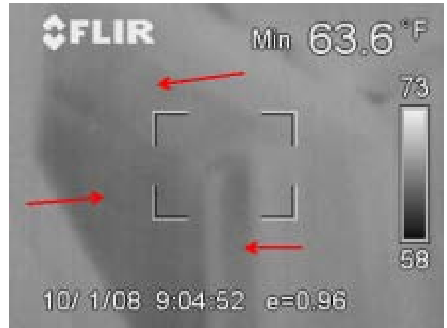
Uninsulated wall and open wall cavity to the outside
