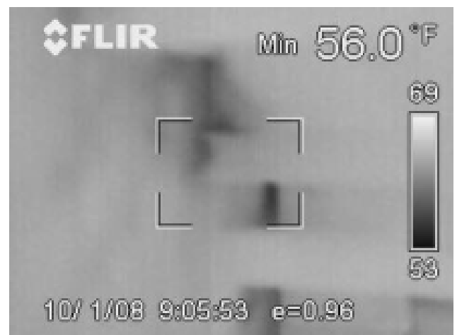
Needs foaming or other sealant
